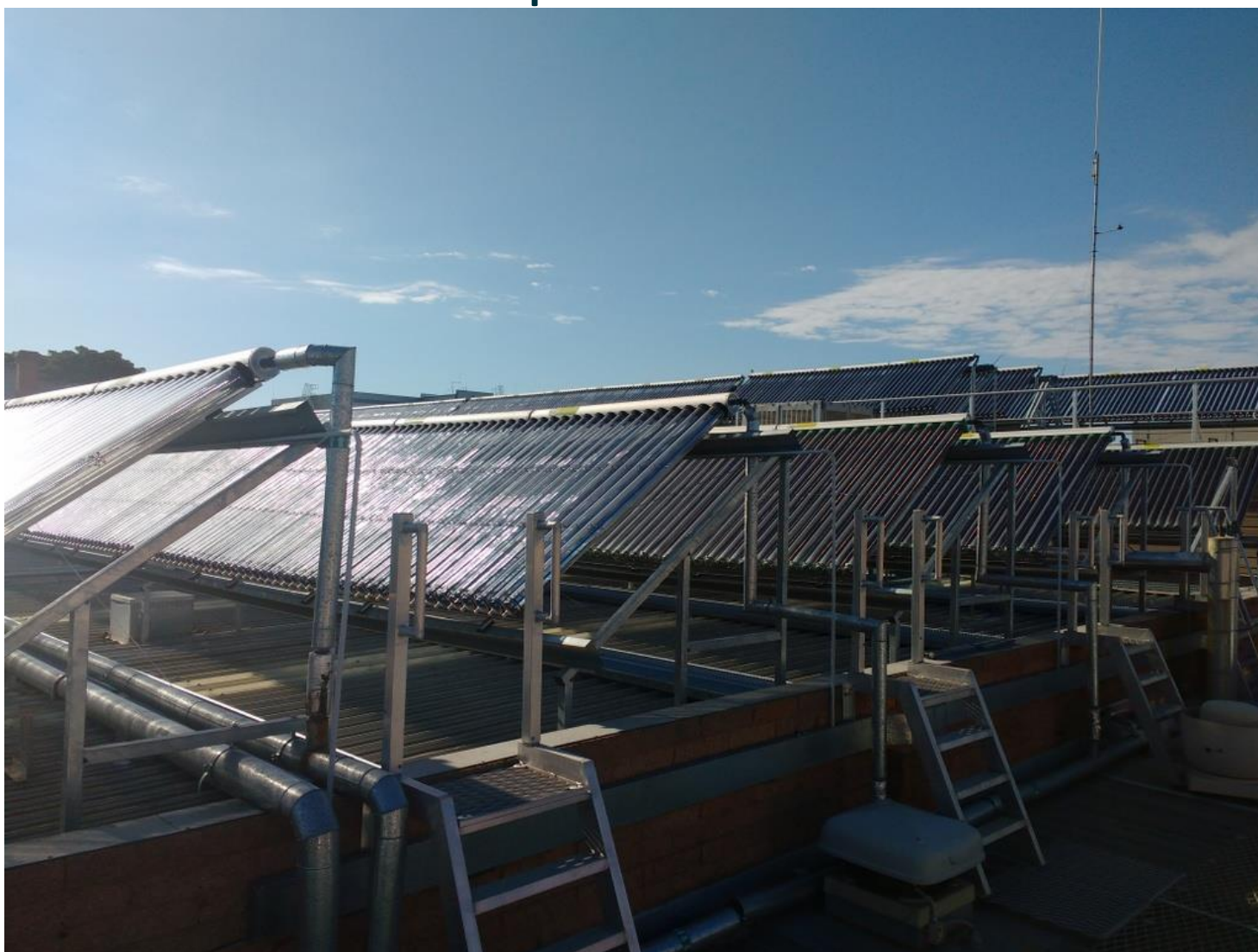
144 collectors ; 500 kW Broad chiller
