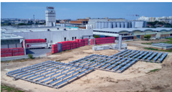
660 m 2 parabolic trough collectors for the Brewery Birra Peroni in Bari, Italy
