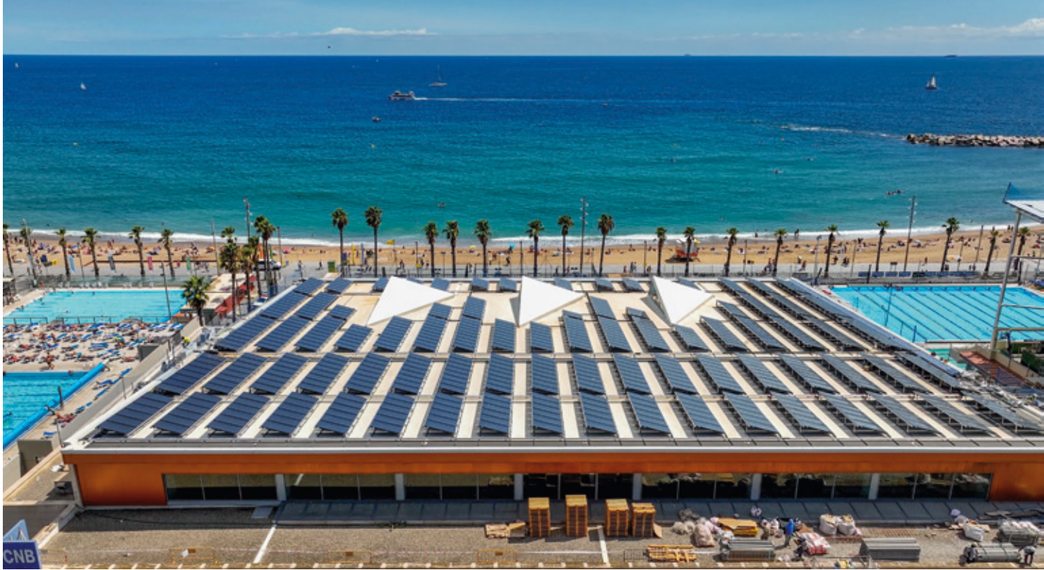
Domestic hot water and swimming pool system with 2,082 m 2 PVT in Barcelona, Spain Photo: Abora Solar, Spain
