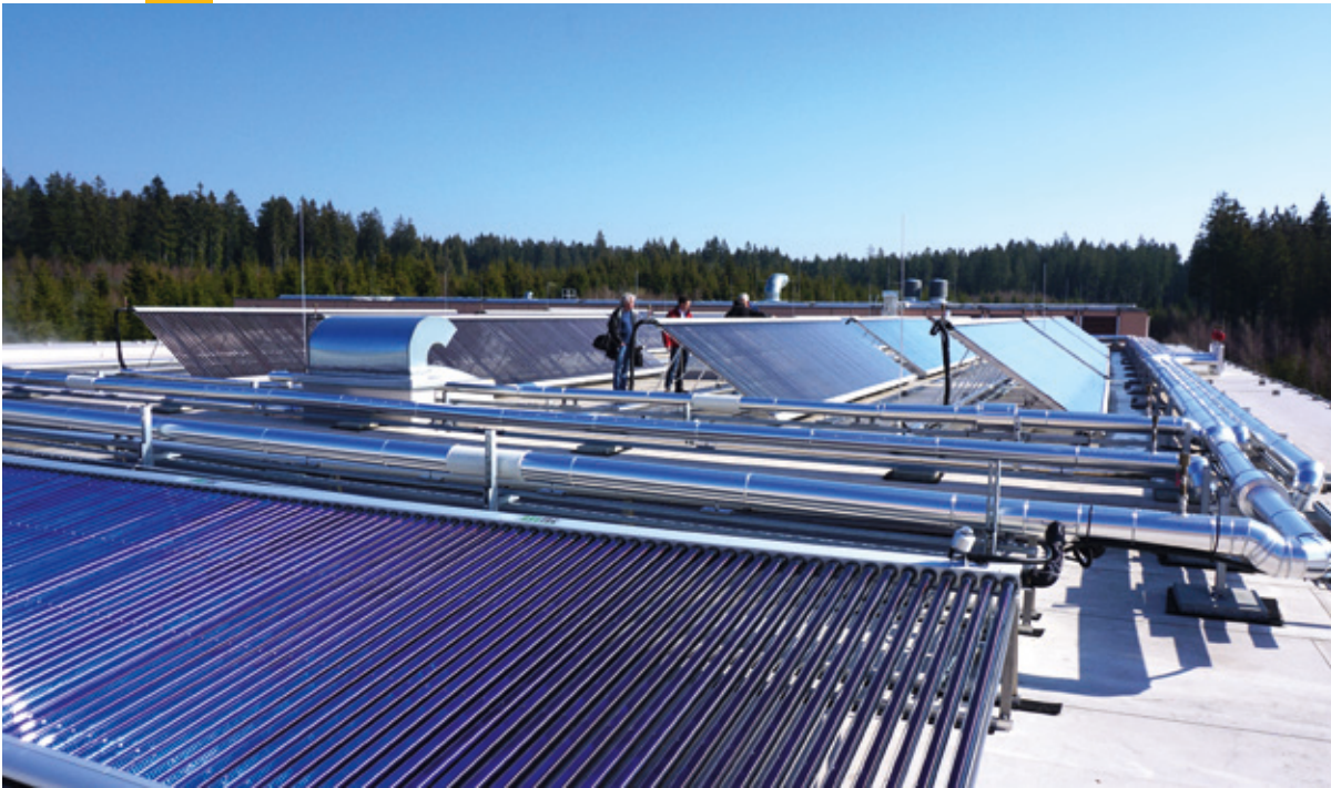
At the Rothaus brewery in Germany, almost 1,000 m 2 of vacuum tube collectors supply the bottle washing machines with heat Photo: Rothaus brewery, Germany
