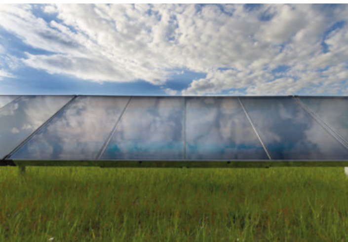
Photo: Savo Solar / Solar Heat Europe
