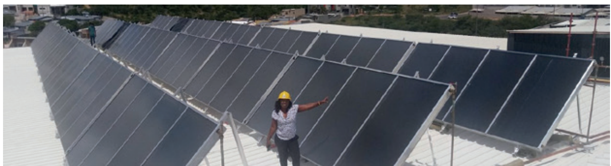
Pumped 210 m 2 flat-plate collector system at the Lady Pohamba hospital in Windhoek, Namibia Photo: Werner Weiss, AEE INTEC
